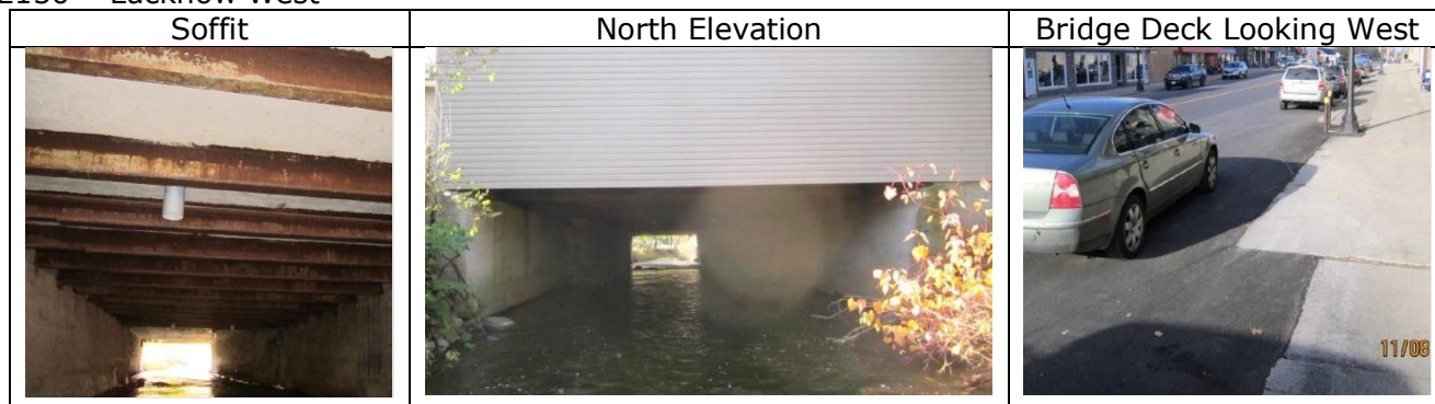
Figure 96 Bridge in Poor Condition (45 BCI)
